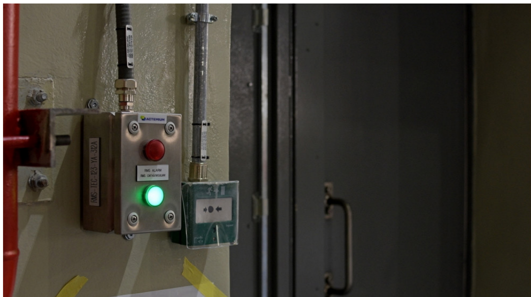
Fig. 1.37 — Testing of the radiation monitoring system
