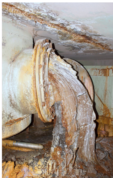
Fig. 2.25 — Brown LFCM in the valve of room 210/7
