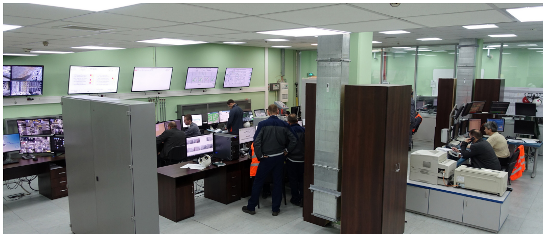
Fig. 1.29 — The unit of the central control panel
