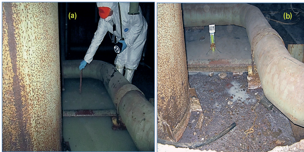
Fig. 3.55 — Radioactive water accumulations in room 012/16: a — September 2016; b — February 2020
