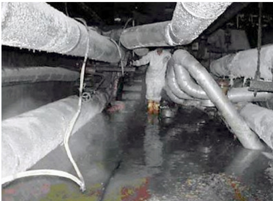
Fig. 3.51 — Radioactive water flowing into the premises of the third power unit of the Chornobyl NPP [113]
